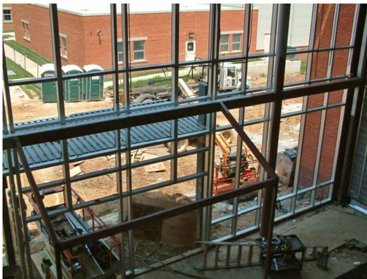
Office of Public Information Work progresses on Carroll Community College's Building No. 4. The classroom suites and dining hall are accented with large windows and cozy niches throughout the 77,000-square-foot space. See page 2 for additional photos.
