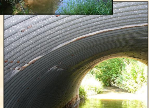
Top photo: end view of the Bixlers Church culverts Bottom photo: looking through the culvert
